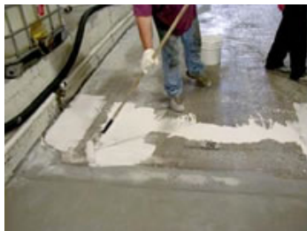
7. Pour appropriate amount of material onto slab and spread evenly with a roller or squeegee.
